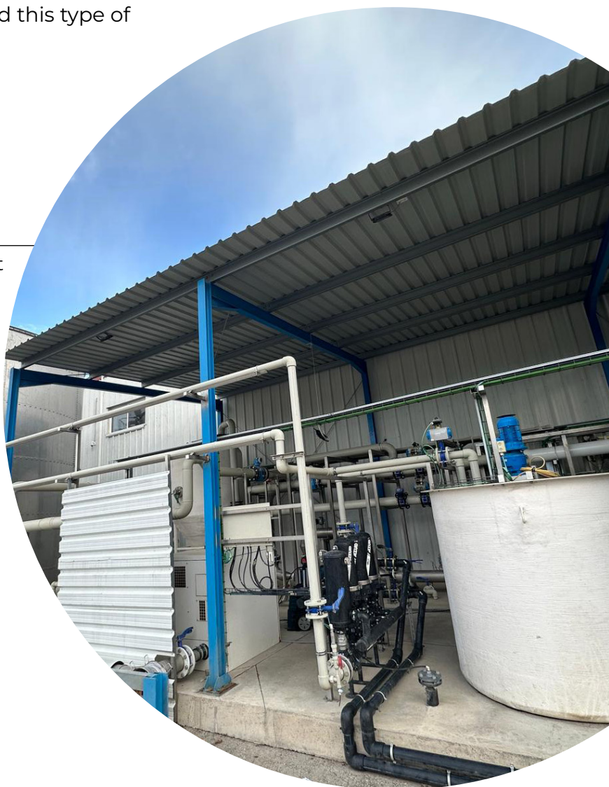
○ Water treatment plant at the Tortosa site
