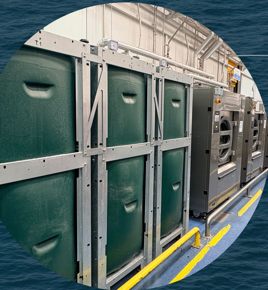
Recovery units on the washing machines at the Valladolid plant
